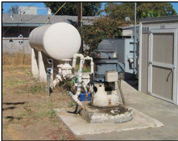
Figure 4.4 Photograph of Well 3
