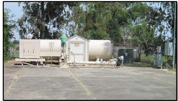
Figure 4.10 Photograph of Well 10
