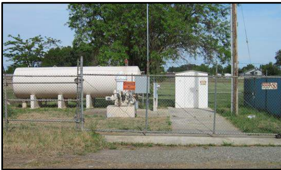
Figure 4.11 Photograph of Well 11
