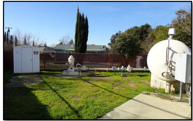
Figure 4.5 Photograph of Well 4
