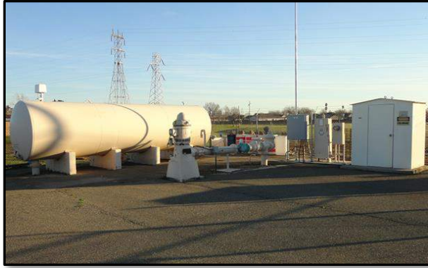
Figure 4.9 Photograph of Well 9
