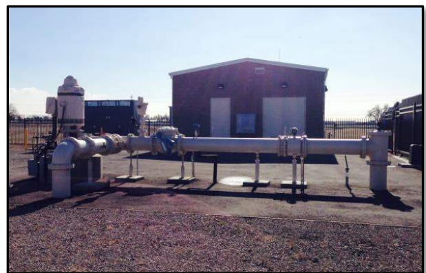
Figure 4.15 Photograph of Well 15
