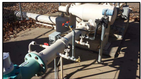
Figure 4.12 Photograph of Well 12
