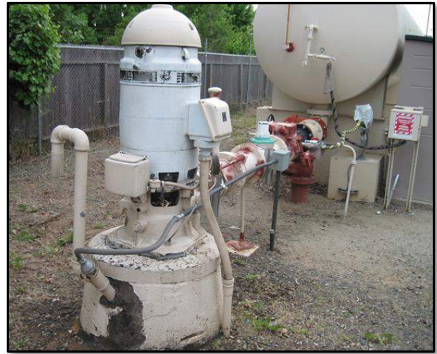
Figure 4.7 Photograph of Well 7
