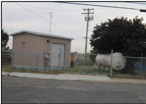
Figure 4.16 Photograph of Elverta Booster Pump Station
